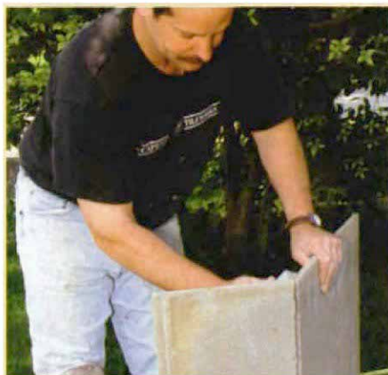
2. Score the back, too. After snapping the cement board along the score line, Meehan cuts through the back of the sheet, like working with wallboard.
