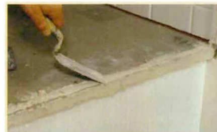
6. Finish edges with thinset. Fiberglass mesh tape and a thin layer of thinset adhesive finish the edges. This substrate is now ready for tile.
